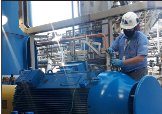
Pulp and Paper Mill looking to enhance reliability of pump motor.
